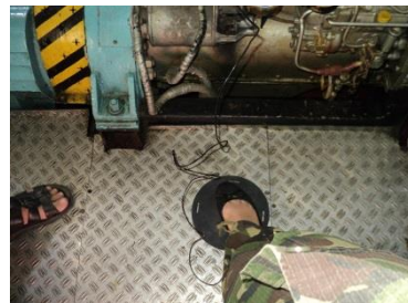
Fig. 7. WBV - engines room
