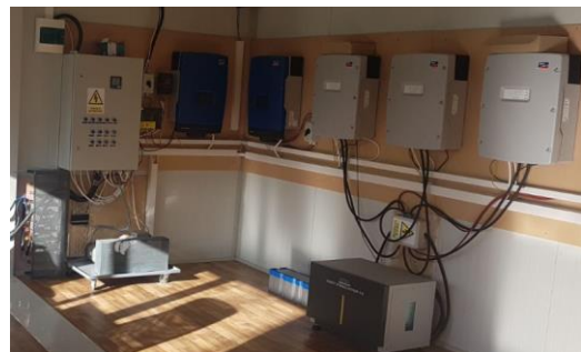
Fig. 5. The three Sunny Island 4.4M-12 off-grid inverters of 3.5kW each, [5]
